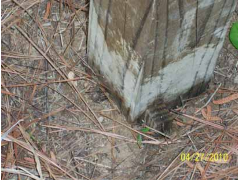
Figure 13. Picture of a treated southern pine 4x4 at ground level in the accelerated plot at Dorman Lake plot with a fungal-infested feeder strip showing on the right face and a second feeder strip barely visible on the left face. The feeder strips are untreated southern pine sticks which were infested at Dorman Lake by being layered with various local decaying woody material and when decay was apparent were placed next to all four faces of the 4x4s in the accelerated plot.
