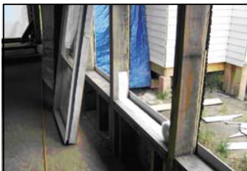
Figure 4 – A borate-treated fibrous strip being fastened to the house framing prior to installation of windows.
