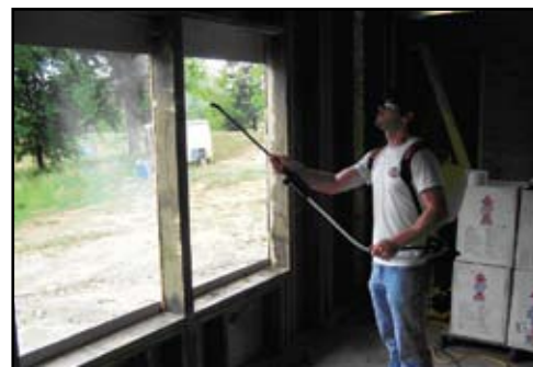
Figure 5 – Framing adjacent to a window opening, and framing/sheath below the opening being sprayed with a water-repellent preservative prior to installation of a window.
