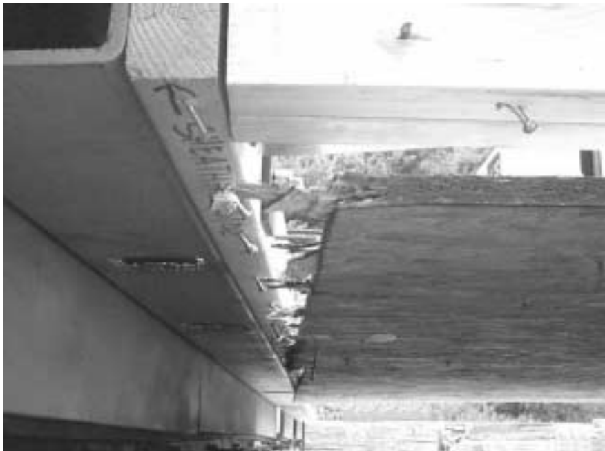
Figure 9. — Typical view of the wall bottom after failure.
